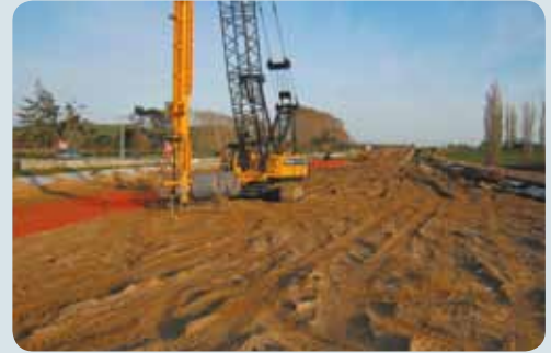
Over 15,000 wicks will be installed alongside SH2 to help drain the water content from the soft soil below.
