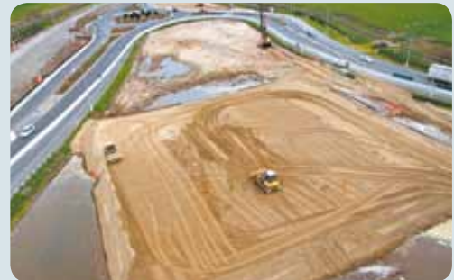
Three trial embankments will be constructed alongside SH2 similar to this one at Domain Road interchange.
